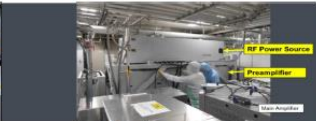
1st Amplifier installation in 2015
