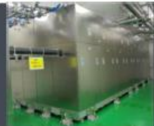
Amplifier system installation in 2016
