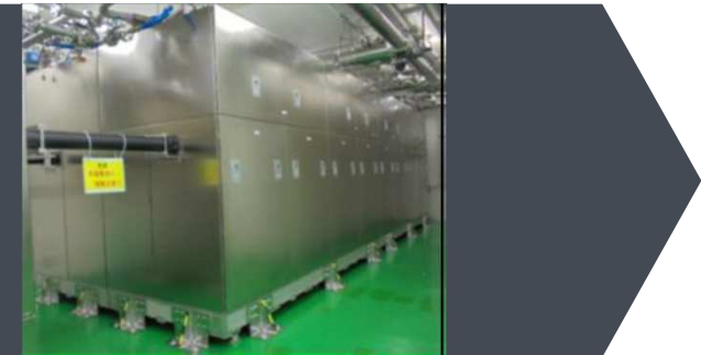
Amplifier system installation in 2016
