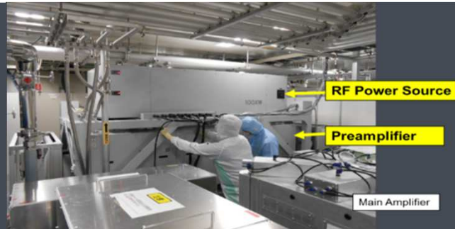
1st Amplifier installation in 2015
